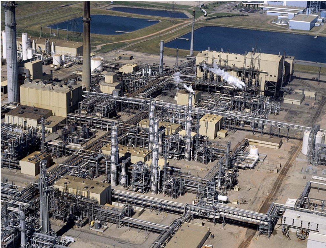
5 Figure 3.15. North Dakota coal gasification plant with 3.3 \text{ MtCO}_2 \text{ yr}^{-1} capture using a cold methanol, physical solvent process (cluster of 4 tall columns in the middle of the picture represent the \text{H}_2\text{S} and \text{CO}_2 capture processes; part of the captured stream is used for EOR with \text{CO}_2 storage in Weyburn, Saskatchewan, Canada).
