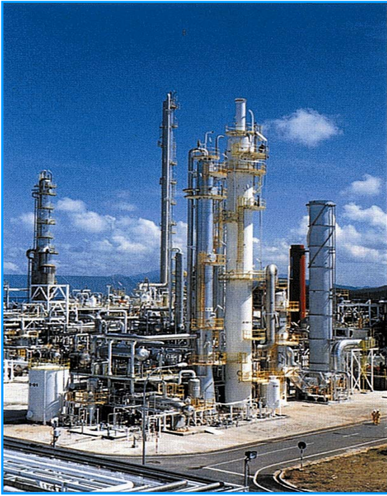
Figure 3.5. CO 2 capture plant in Malaysia using a 200 tonne d -1 KEPCO/MHI chemical solvent process (Courtesy of Mitsubishi).
